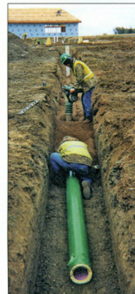
Corey O'Laughlin (foreground) and Kyle McNallan install 6-inch insulated Insul-Seal PVC pipe from the building to the septic tank.
