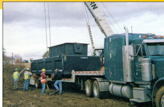
Gary Thill, operator for Modern Crane of La Crosse, Wis., prepares to lift the bottom half of a 10,000-gallon tank with the HighStrengthFAST unit inside. (Photos courtesy of O'Laughlin Plumbing and Heating)
