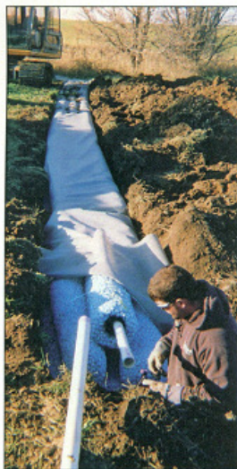
Corey O'Laughlin glues 4-inch Schedule 40 perforated corrugated PVC pipe together for the pressure distribution system. The pipe is inside the Smart-Rock geosynthetic aggregate drainage tubes.
