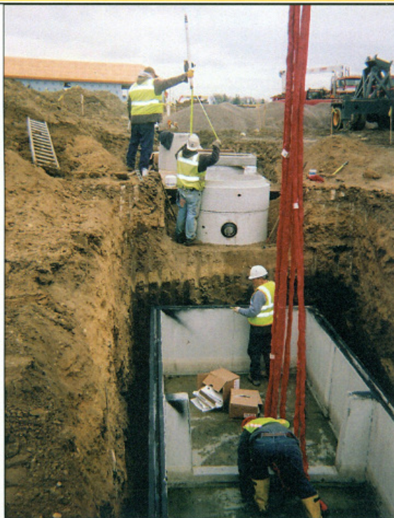
In the background, Wayne Hornberg (left) and Corey O'Laughlin set grades for the manhole covers. Steve Mader (bending over) disconnects the crane from the 6,000-gallon surge tank.
